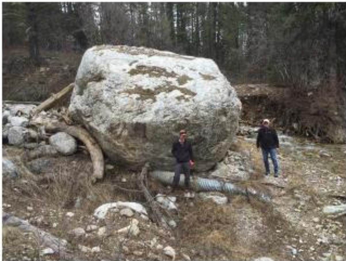
Photo 23 Jensen Creek Diversion Structure Crushed by a Boulder During a Debris Flow.
