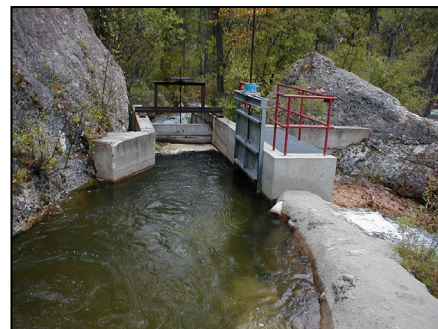
Mead & Coffeen crossover diversion structure (left) next to fish hatchery diversion (right)
