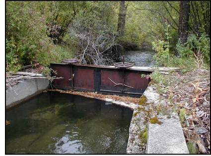
Piney & Cruse primary headgate
