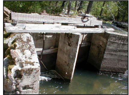
Mountain Supply Ditch Headgate
