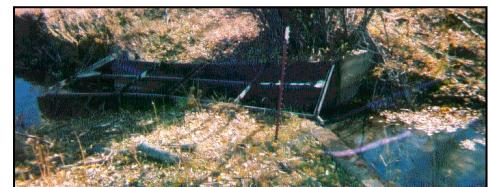
Penrose Ditch at French Creek flume
