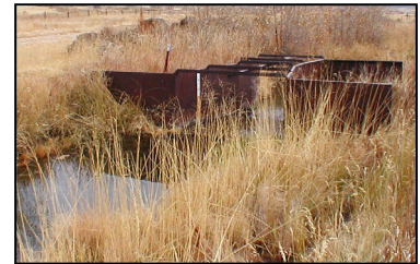
Moreton Ditch flume
