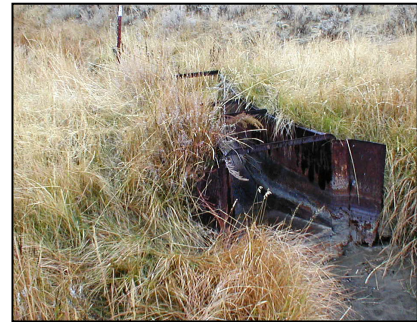
Cook Ditch Flume
