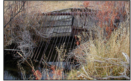
North Fork Diversion Headgate
