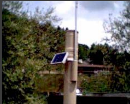
Automated Rain Gages
