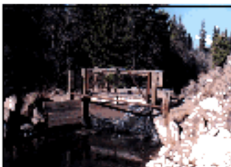
Hilliard East Fork diversion structure
